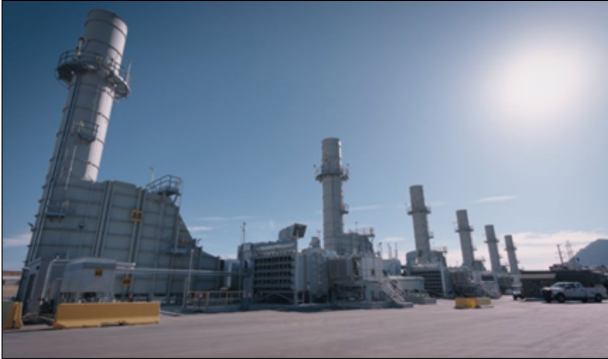
Figure A- 3: South Plant Aeroderivative Generators
