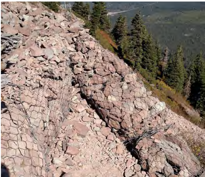
Figure 4–46. Place rock tightly to avoid failure. This failing gabion was constructed with inadequately sized material and without sufficient batter. Shasta-Trinity National Forest, California. USDA photo.
