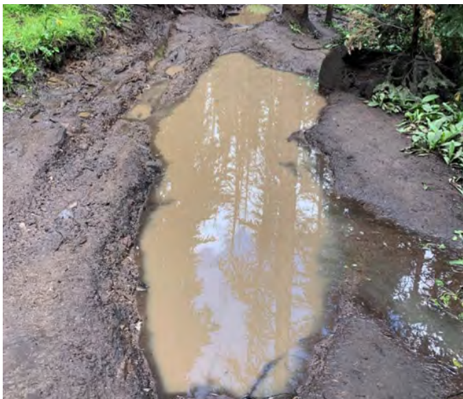
Figure 4–1. Water pools in ruts created when the trail is saturated. Solutions for this include more effectively removing water from the trail, installing a forced uphill undulation, or hardening sections where rerouting isn’t possible and draining is not effective. USDA photo.
