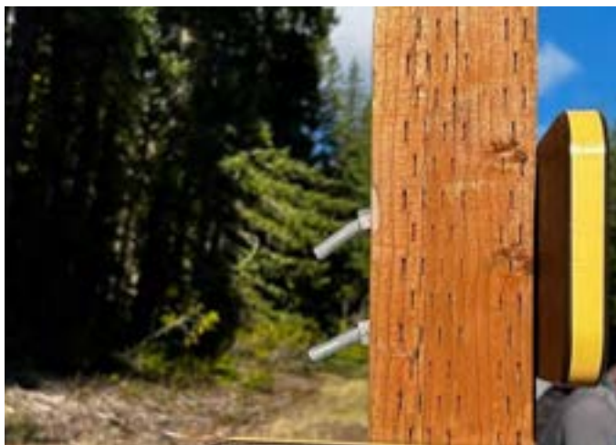
Figure 3-1. Bending the ends of through bolts can help prevent sign theft. Mt. Hood National Forest, Oregon. USDA photo by Meckenzie Helmandollar-Powell.
