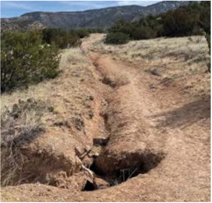
Figure 2–6. Water has concentrated along the berm, causing erosion. Cibola National Forest, New Mexico. USDA photo by Kerry Wood.
