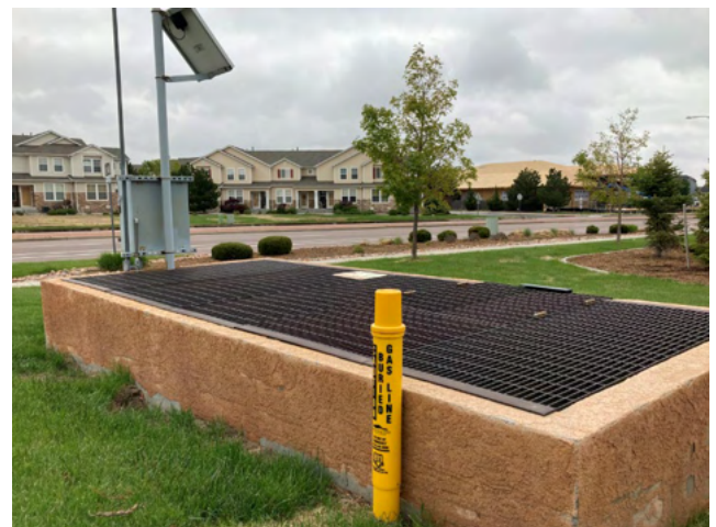
Natural gas regulator station.
