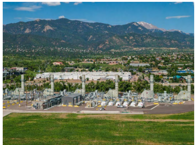
Natural Gas Generating Units at South Plant.
