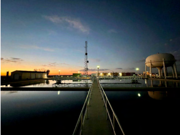
Sedimentation basins at Fountain Valley Authority Water Treatment Plant.
