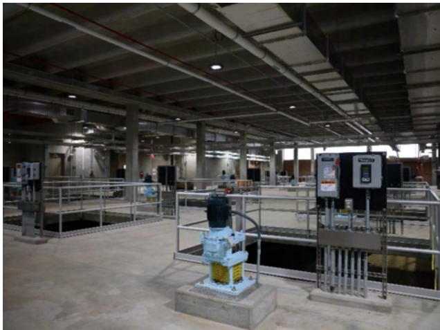
Coagulation and flocculation basins at the Phillip H. Tollefson Water Treatment Plant.
