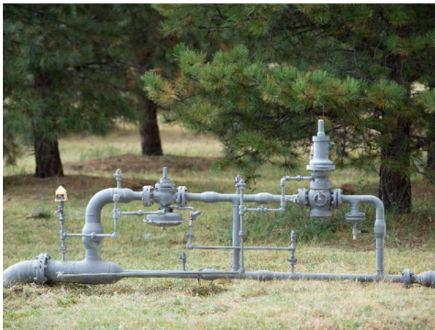
Natural gas gate station.
