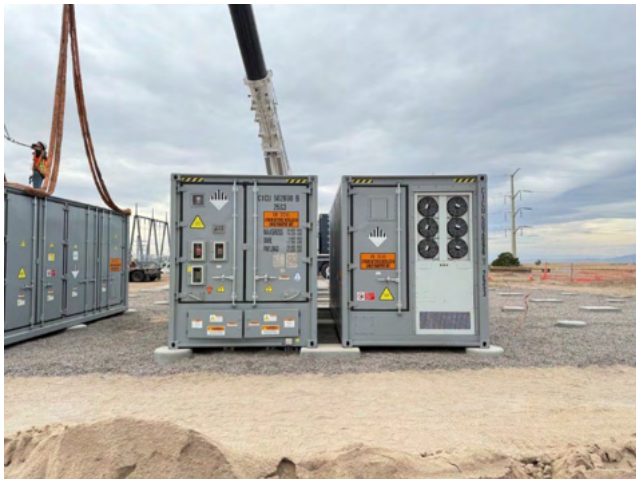
Lithium-ion batteries at the Jackson Fuller Substation in northeastern Colorado Springs.
