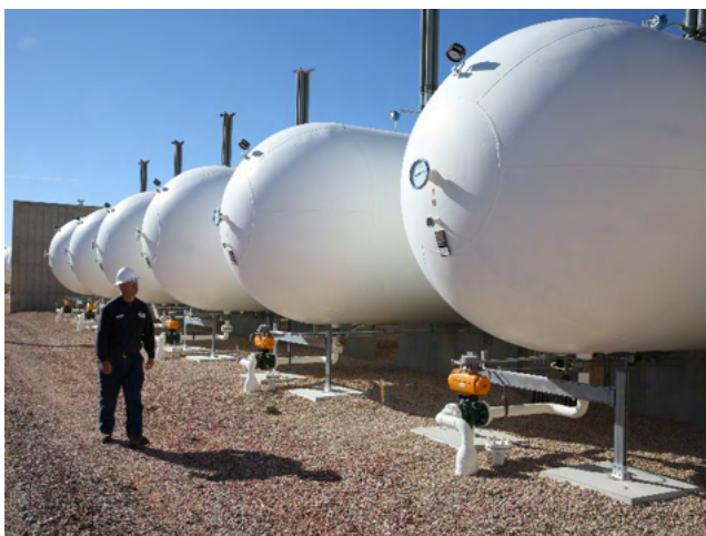
Employee walking by Gas Propane Air Plant tanks.
